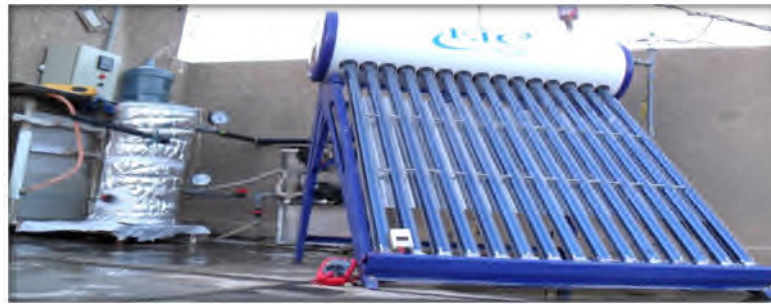
Figure (2) Set up of the heat exchanger in solar energy system
