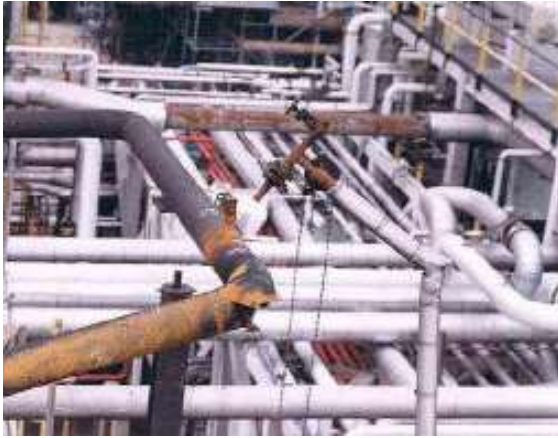
Figure 1: Piping systems in oil industry showing erosion occurs in elbows.
