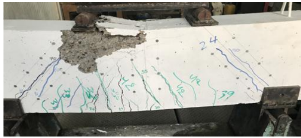
Plate 2: Cracks pattern of beam C-B1
