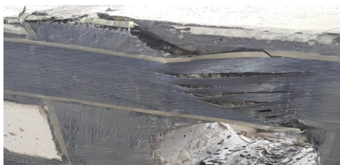
Plate 8: Tearing of CFRP strips
