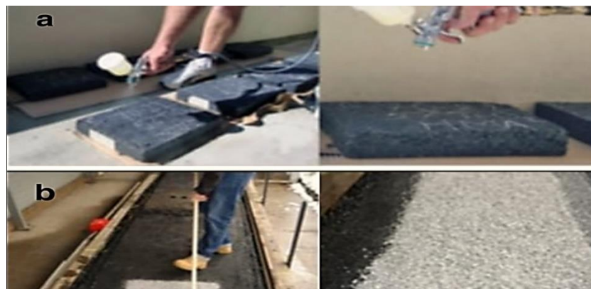
Figure 4: (a) The TiO 2 solution spraying process (b) the painting process of TiO 2 solution [43]
