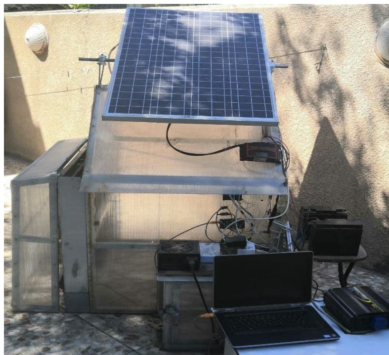
Figure 4: Control system with the greenhouse
