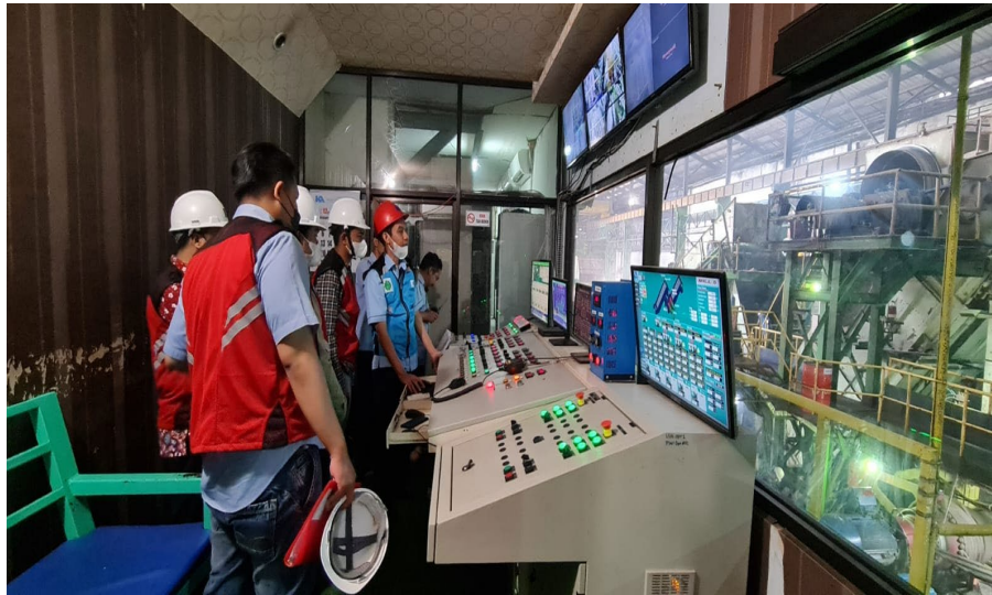
Figure 3: Retrieval of motor and turbine data in the control system
