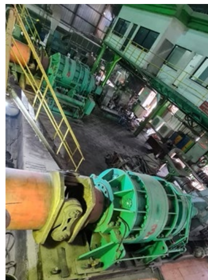
Figure 2: Steam turbines at mills 3 and 4
