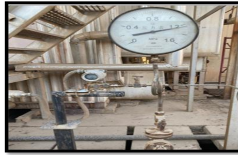
Figure 4: The gauge of drum pressure in the (Al-Quds power plant).
