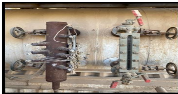
Figure 5: The gauge of the water level in the (Al-Quds power plant).
