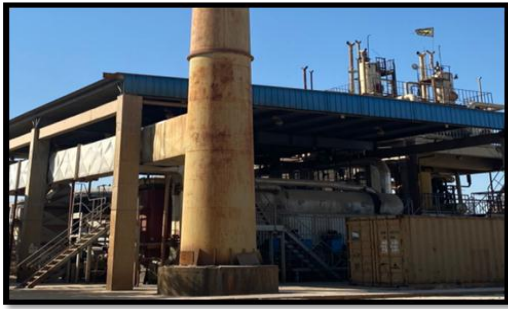
Figure 3: The water tube boiler in (Al-Quds power plant) Baghdad / Iraq.
